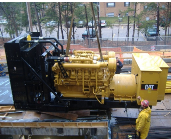
Figure 5: Image of Generator
